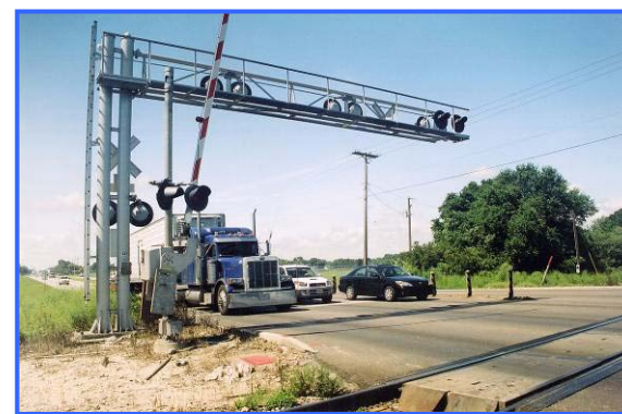
Crossing signal and gates on Park Road at US 92 in Plant City.
